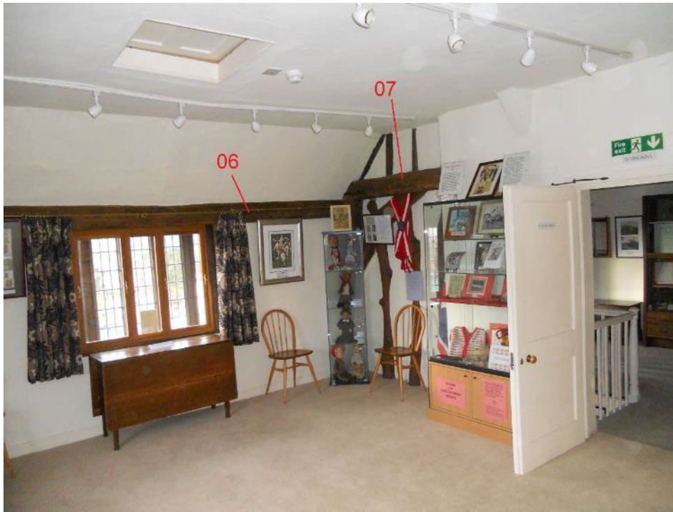
Figure 5: Photograph of the west side of the second floor, looking west, showing timbers sampled (photograph Martin Bridge)
