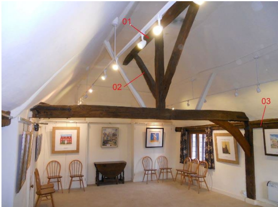
Figure 3: Photograph of the east side of the second floor looking north, showing the timbers sampled for dendrochronology (photograph Martin Bridge)
