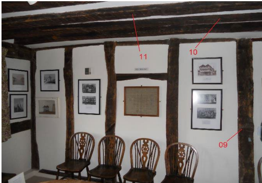
Figure 7: Photograph of the wall separating the Small Room and the Council Chamber on the first floor, showing some of the timbers sampled for dendrochronology (photograph Martin Bridge)
