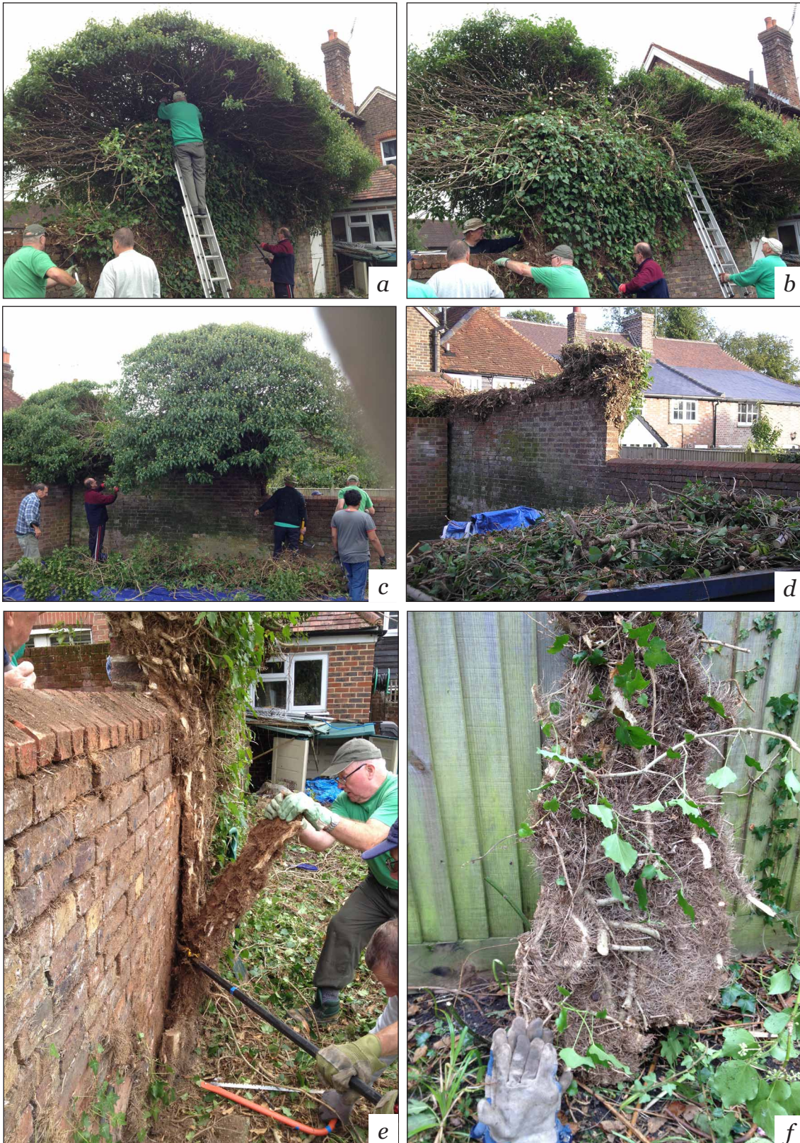
Figure 4-9. Spreading flowering stems were first removed, followed by vertical foliage covering the wall. The dense mat of stems was sawn and prised off using a crow-bar were possible.
