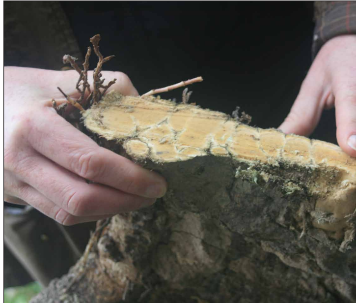
(b) Mass of compressed ivy stems removed from the base of the crack.
