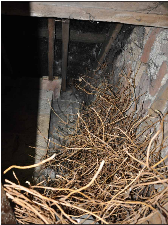
(c) Mass of ivy stems within the porch roof space.
