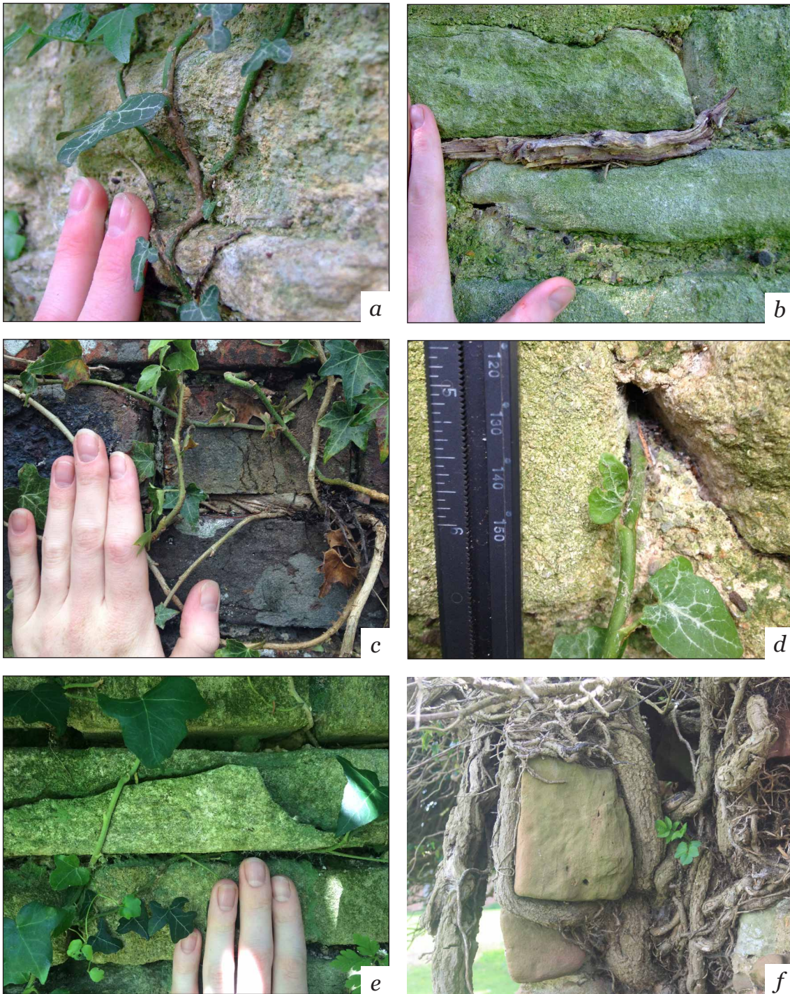
Figure 2-11. Examples of typical growth responses of juvenile ivy stems to different kinds of wall features: (a) stems closely follow the contours of shallow mortar joints; (b) thickened stems in joints are difficult to remove completely; (c) stem thickening within joints may cause stress cracking of adjacent masonry blocks; (d) stems entering small holes can grow into internal void space (where this already exists) as they cannot turn and exit; (e) stems growing in and around surface deterioration can aid detachment of loose pieces of stone; (f) stems growing through walls (from one side to another) and around masonry blocks can cause considerable damage, but may also support poor condition walls. (f ©Alan Cathersides)
