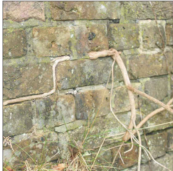
(b) Ivy stems following eroded mortar lines at Dover Western Heights.
