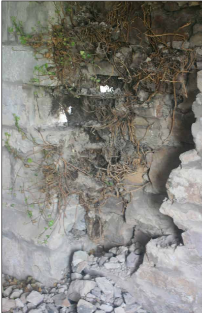
(a) Mass of ivy stems and roots within the core after removal of several layers of internal stone.
