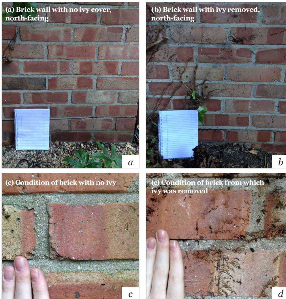
Figure 4-2. Areas of brickwork on which surface moisture readings were taken: (a) and (c) an area without any previous ivy cover; (b) and (d) adjacent area from which a complete cover of ivy has been removed.
