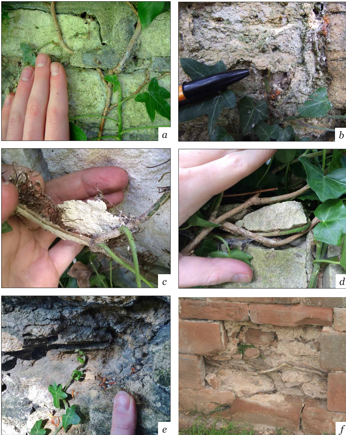
Figure 2-12. Ivy stems interacting with existing deterioration features: (a) growth under loosened pointing repairs (Holywell Cemetery, Oxford); (b) penetration into badly deteriorating and friable limestone (Holywell Cemetery, Oxford); (c) aerial rootlet attachment to spalling limestone (Wytham Woods test walls); (d) shoots growing between a fractured limestone block (present before colonisation and possibly caused by frost damage, Wytham Woods test walls); (e) stem growth into, around, and out of larger voids; (f) stems growing into, thorough and out of walls can cause serious damage to walls (Maxstoke Priory, Warwickshire). (f ©Alan Cathersides)
