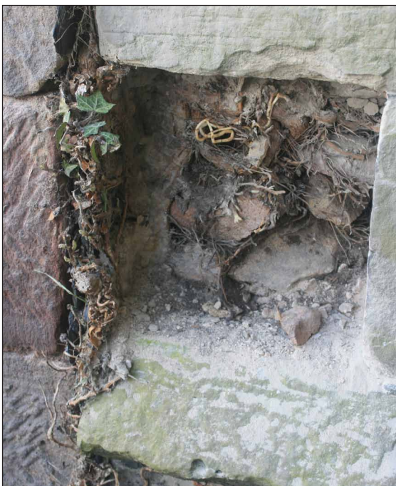
(c) Initial removal of a single external stone revealed ivy stems and roots within the wall core.
