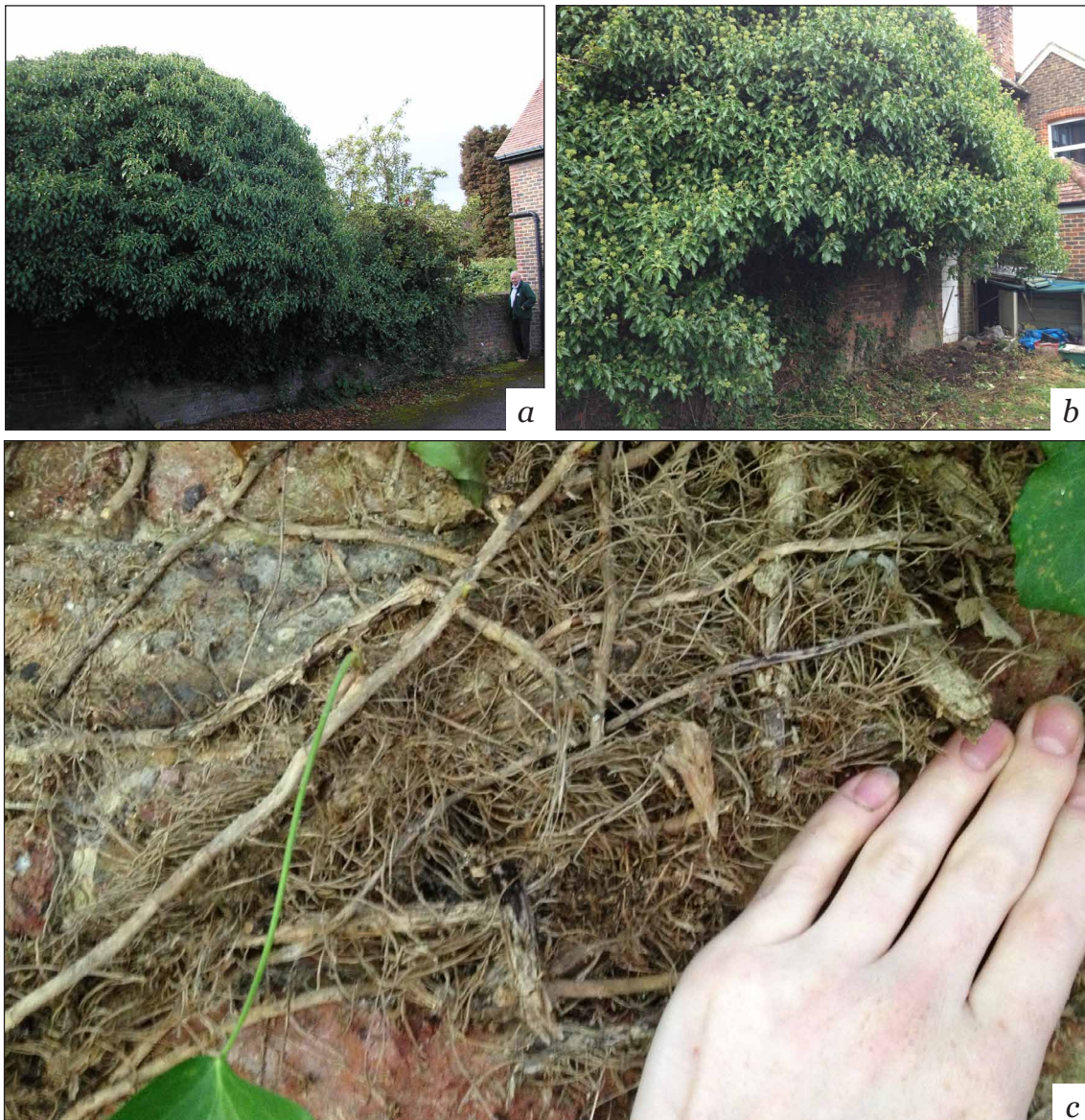
Figure 4-8. Ivy canopy prior to removal (a) north-facing side of the wall; (b) south-facing side of the wall (c) mat of stems growing against the wall surface. Warnham, 2014.
