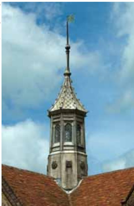
The central cupola or lantern added c.1885, to the designs of the architect, Richard Hussey
