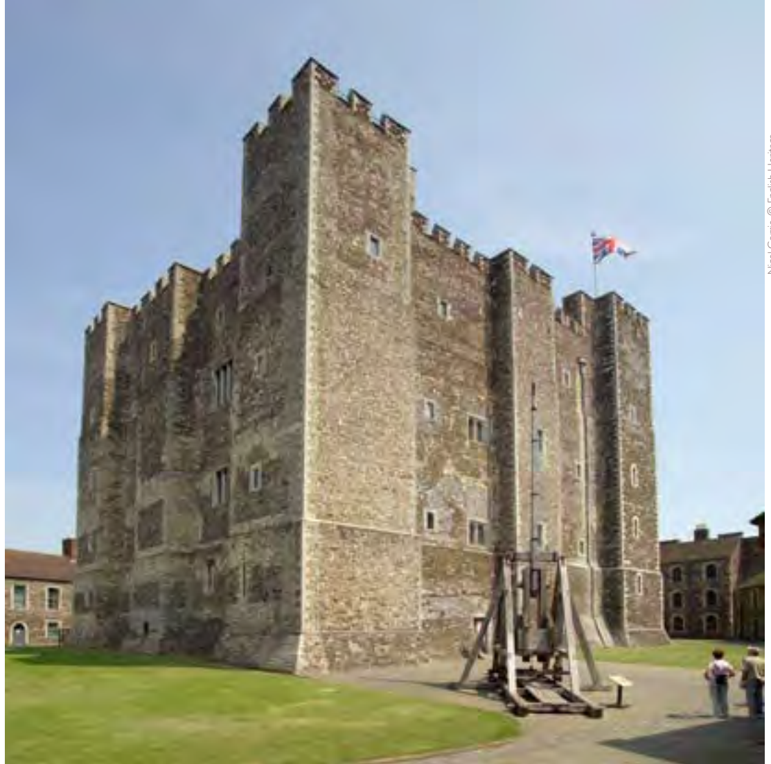
Fig 4: The SW elevation of the Great Tower showing extensive 19th-century re-facing. Though there are clearly two styles at work here, they are likely to date to the same phase of restoration
