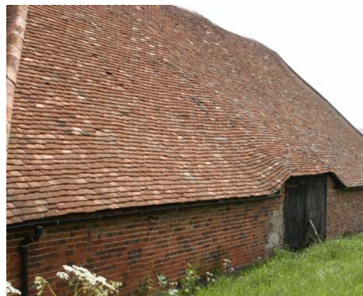
Large expanse of roof of a brick aisled barn. Plain clay tile roof.
