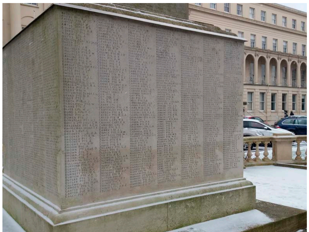
Figure 24: Cheltenham war memorial in Gloucestershire has more than 1,200 men commemorated on it. Each inscription name was originally carved and infilled with mortar. A discreet stainless steel flashing was installed, which seems to have minimised the run-off.
