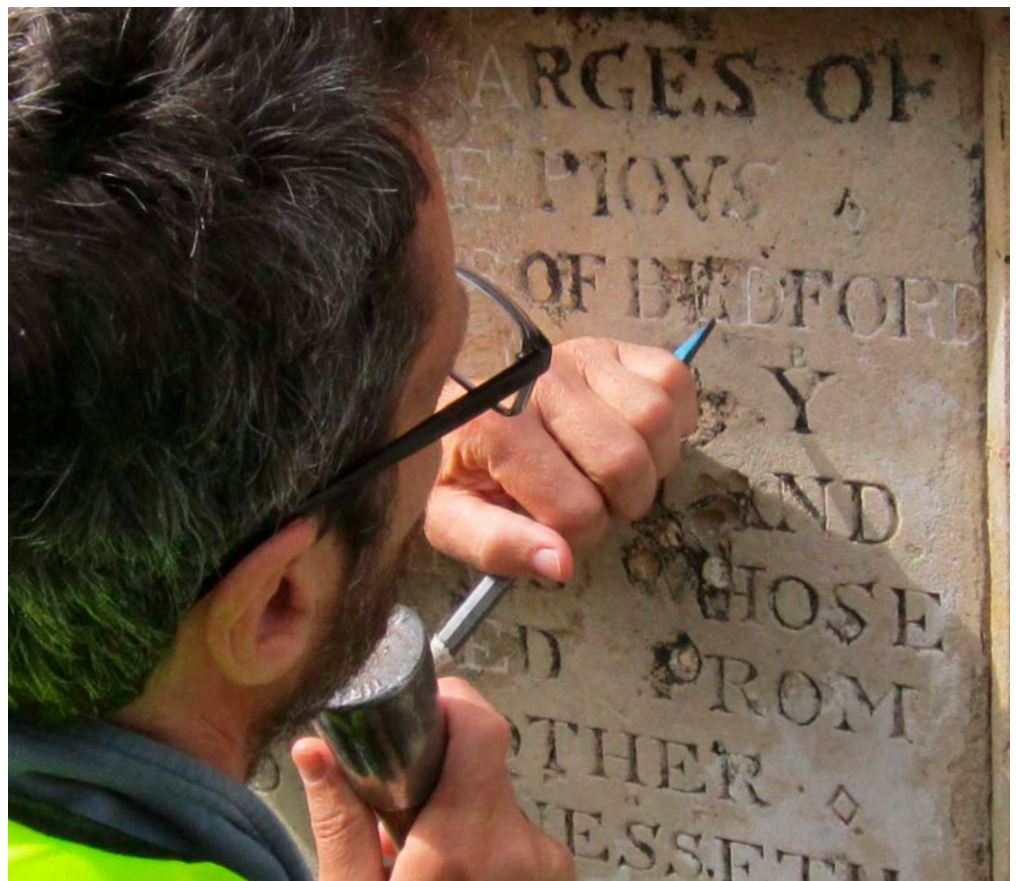
Figure 28: An experienced letter cutter can sharpen the inscription on a deteriorated stone panel to improve its legibility.
