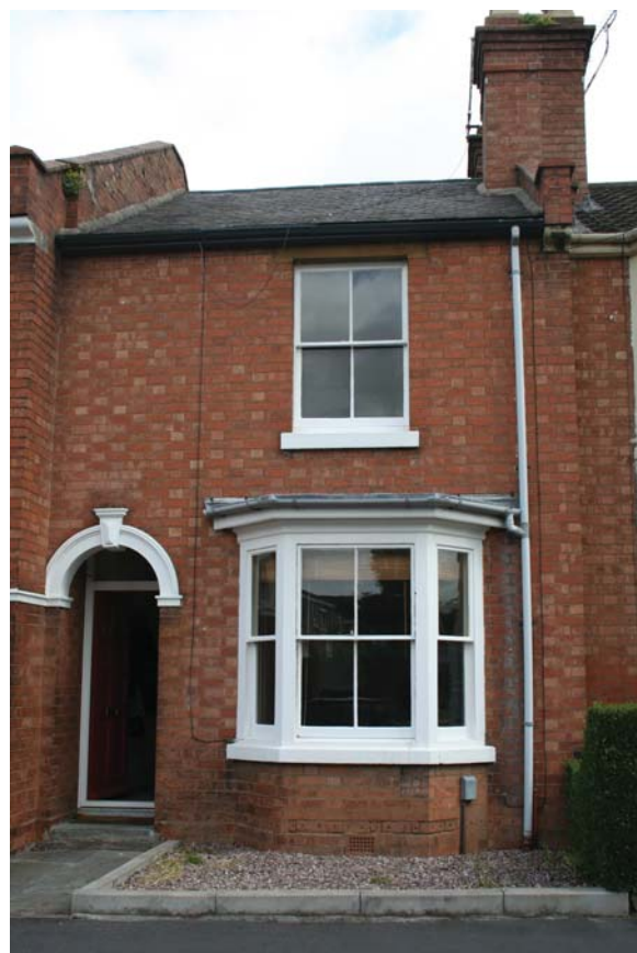
The original windows on this terraced house have been draught-proofed. An air-pressure test showed that this was more effective than that found in 90 per cent of today's new buildings. © English Heritage
