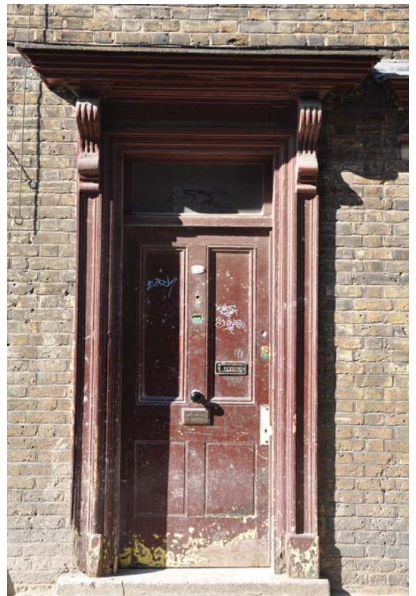
Simple elements, such as this door in Princelet Street, Spitalfields, can be important contributors to the character of conservation areas. © Gareth Wilson
