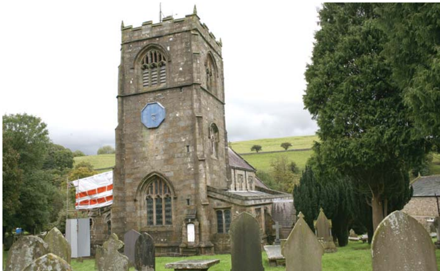
Catastrophic roof collapse or well-protected repair in progress?
