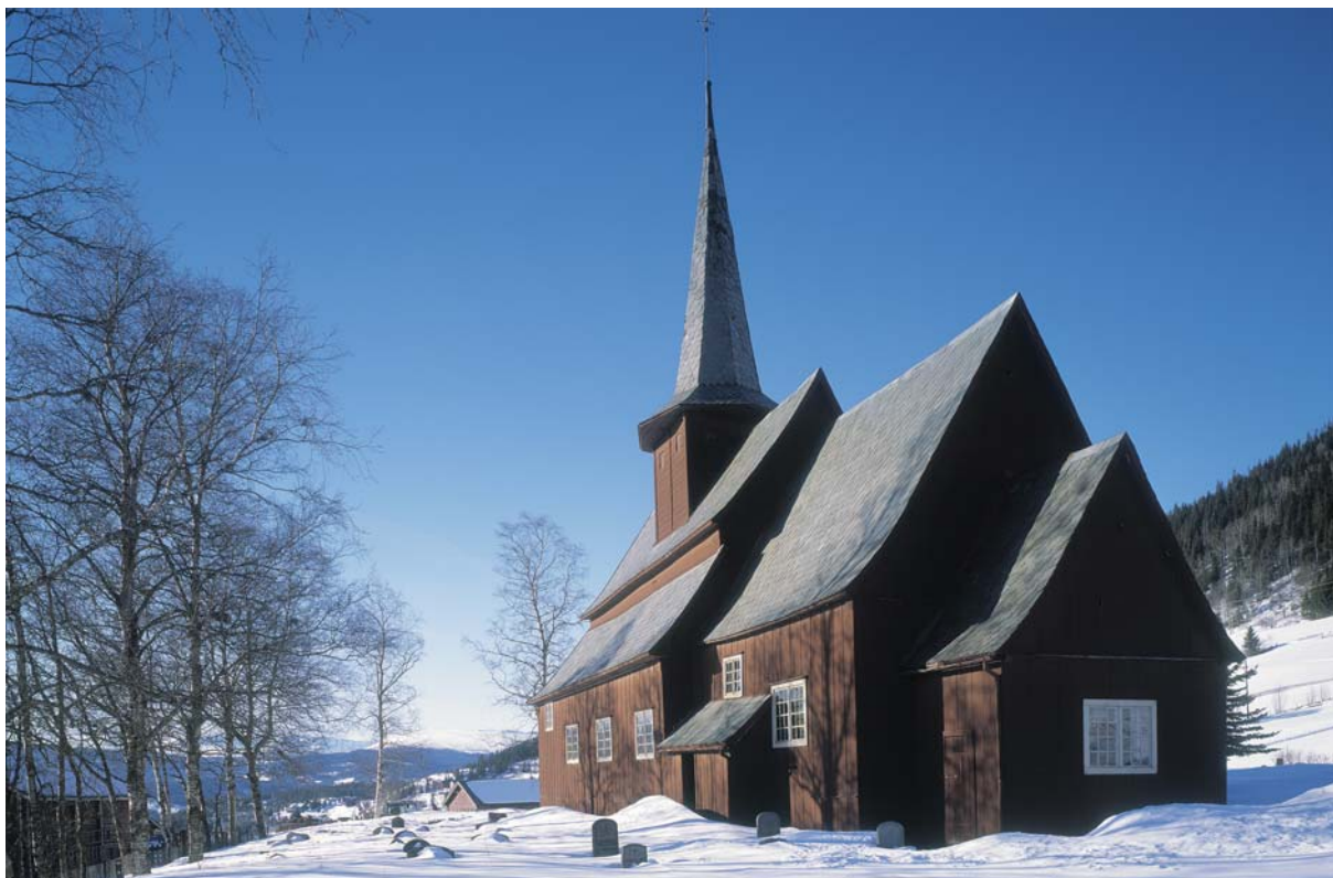
The wooden Hegge stave church, in Valdres. After more than 800 years, the church still is the local centre of Christian worship. The building has had some alterations and restoration, but regular maintenance and care has made it stand up against the wear and tear of time.
