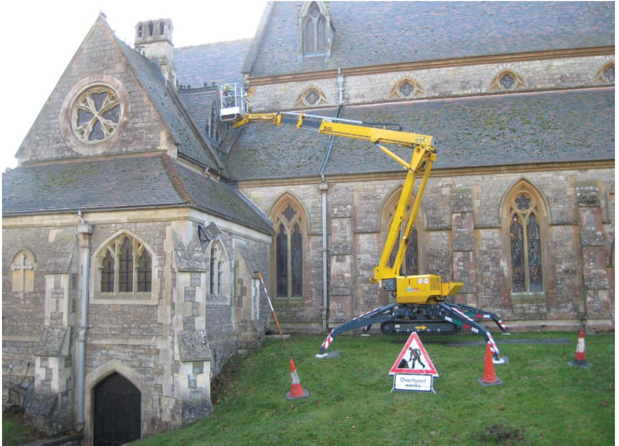
Gutter clearance in action at a church in Gloucestershire. Specialist equipment is often needed to carry out such work safely and efficiently, particularly on large and complex places of worship. © SPAB
