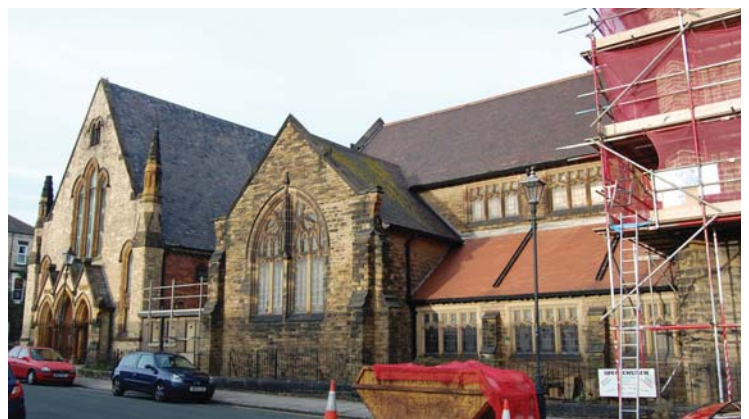
Saltburn-by-the-Sea Methodist Church, Cleveland, during recent repairs to the tower and spire carried out with a grant of £63,000. © English Heritage
