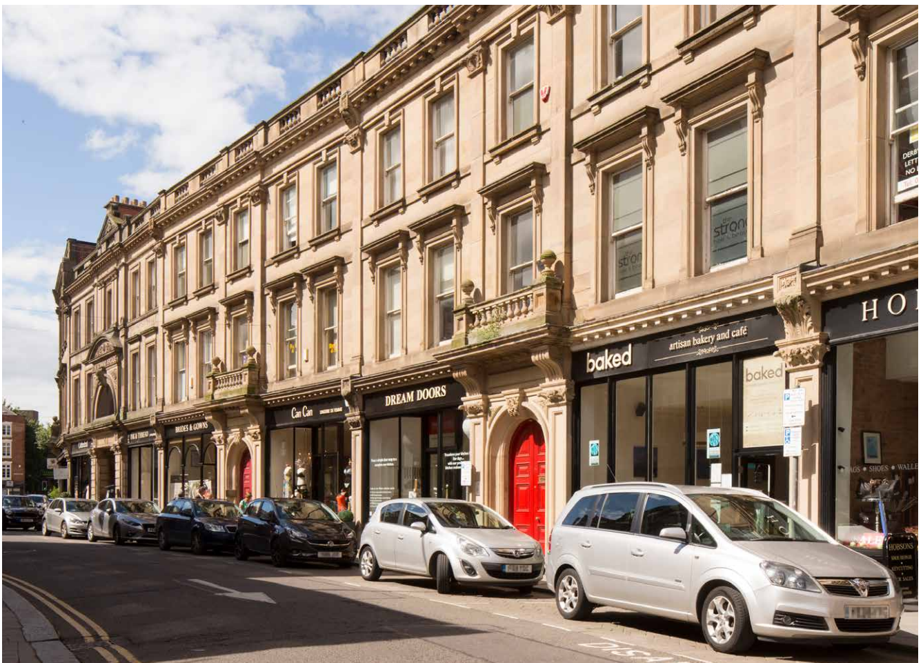
Repair and reinstatement of the historic shop fronts in Derby. © Historic England
