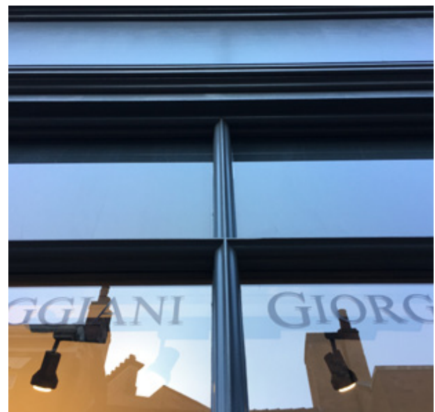
28 Sadler Gate: The project officer worked closely with the contractor to ensure a high quality 'lamb's tongue' finish to the glazing bars.
