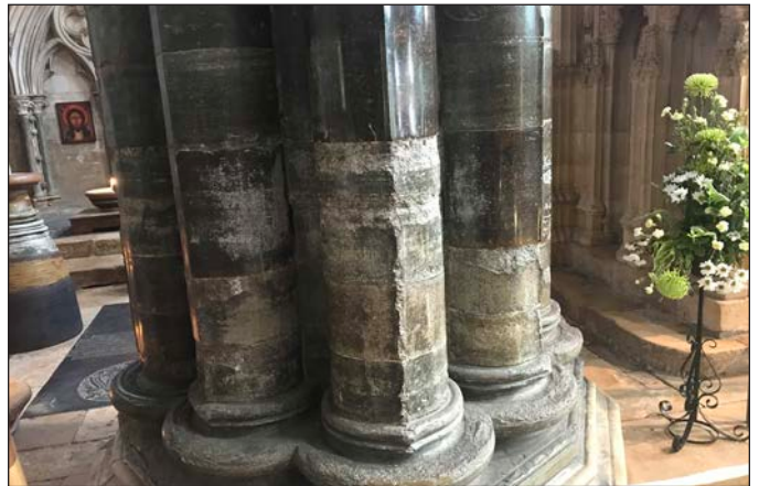
Low level decay on a Purbeck Marble column at Lincoln Cathedral
