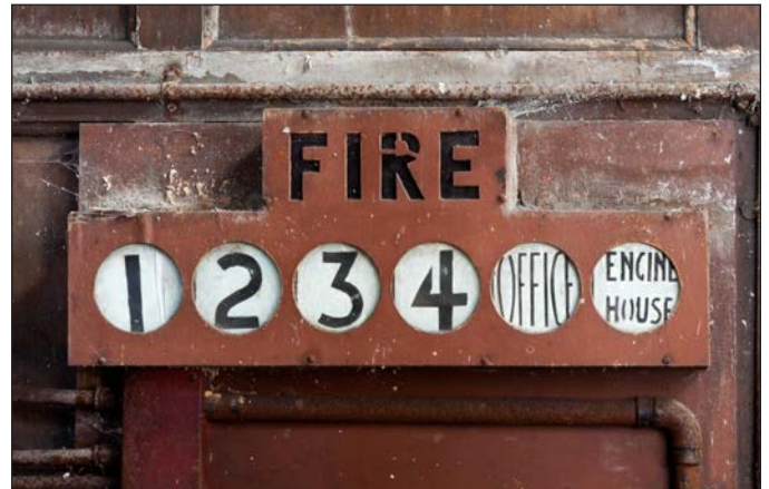
The old fire alarm panel at the Waterloo Mills, Bradford
